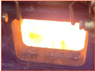
17.4.23. Newheat at Pumphouse 1200 deg.C
