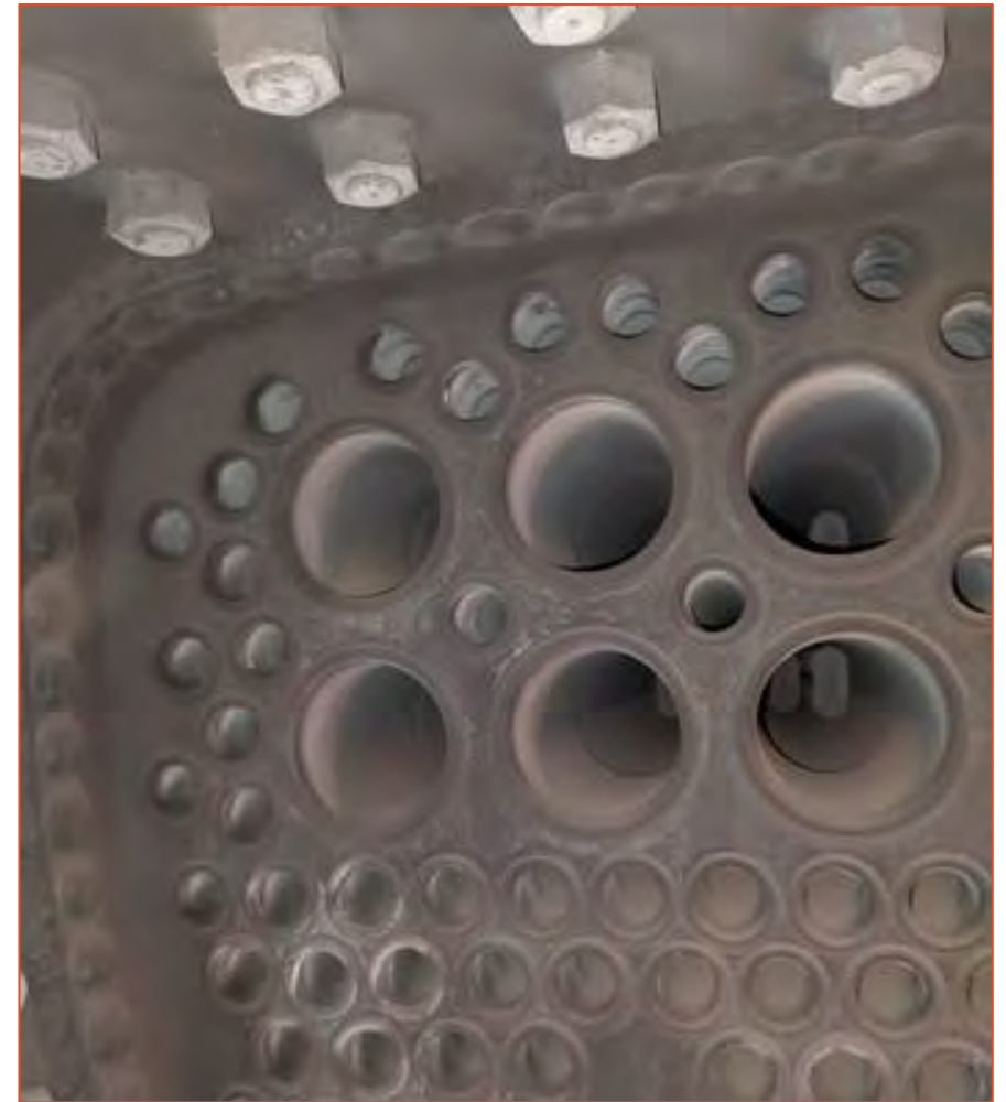
Firebox Tubeplate with low chlorine Wildfire
