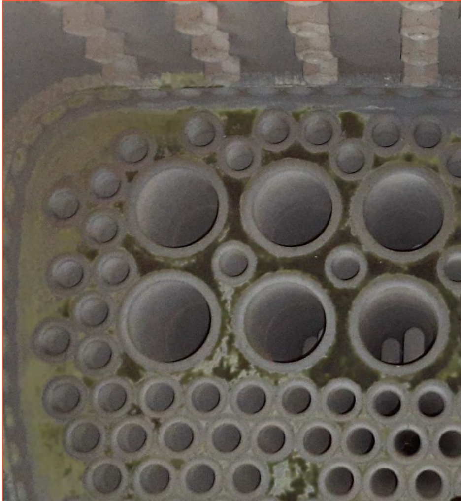
Firebox Tubeplate with high chlorine HB3
