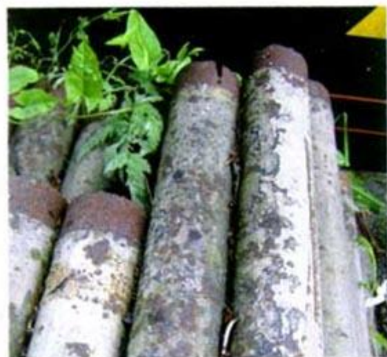
These tubes show the classic problems of scaling (the grey/white deposits) and corrosion. MARTYN BANE.
