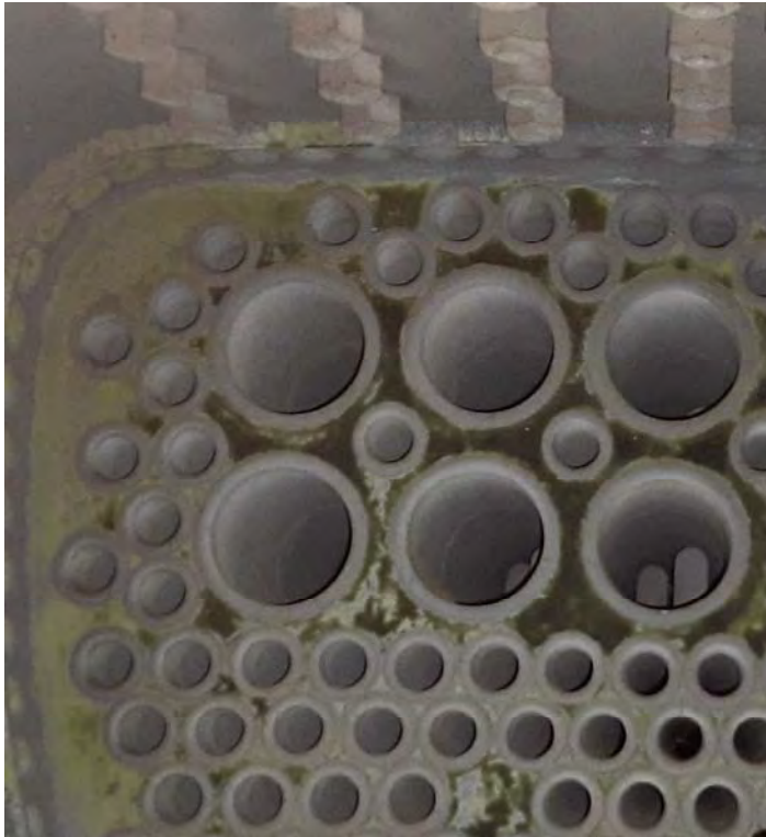
Firebox Tubeplate with high chlorine HB3
