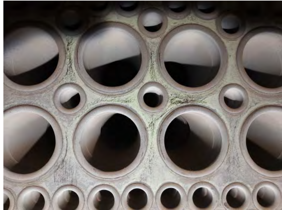
Close up - Firebox Tubeplate
