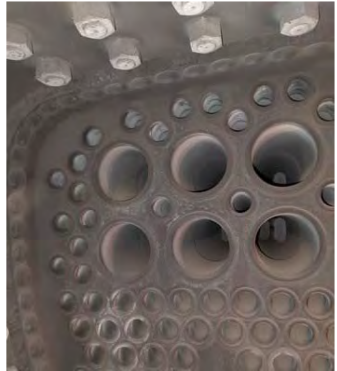
Firebox Tubeplate with low chlorine Wildfire
